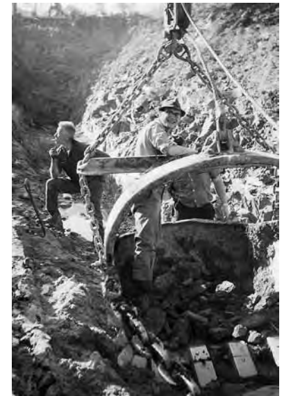
STANDING IN THE BUCKET OF THE DRAGLINE JUST AFTER IT HAD COMPLETED THE TRENCH THAT EXPOSED THE KIDD CREEK OREBODY FOR THE FIRST TIME.
